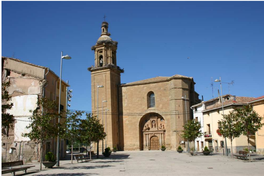
Figure 1 - Santa María la Blanca's church and its leaning bell tower
