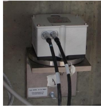
Figure 3. Digital inclinometer enclosure deployed on the cap of pier M6
