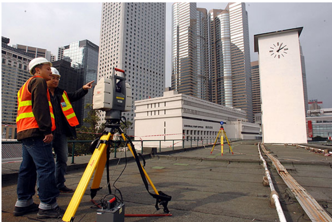
Fig 3. The 3D laser scanning system Leica HDS3000 at the Old Star Ferry Pier
