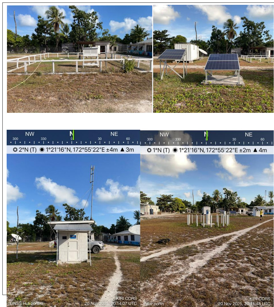
Figure 3: Fenced weather station (top left), solar panels for GNSS hut (top right), GNSS hut (bottom left); and KIRI CORS monument and antenna (bottom right)
