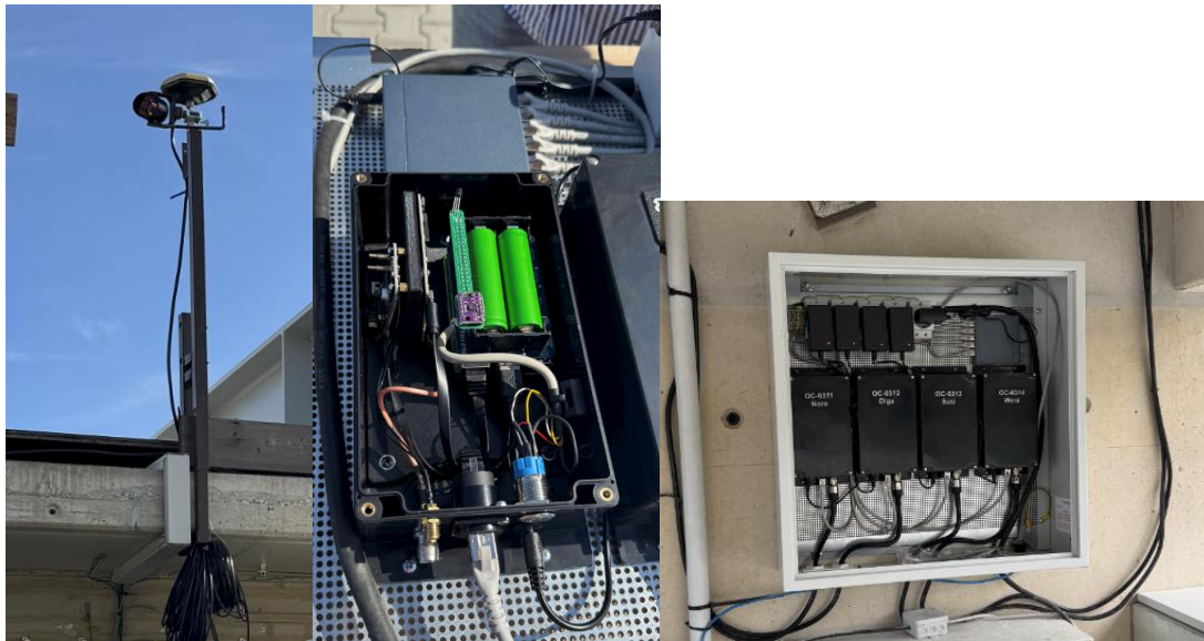
Antenna, data logger (individual units) Equipment cabinet housing the data logger units
